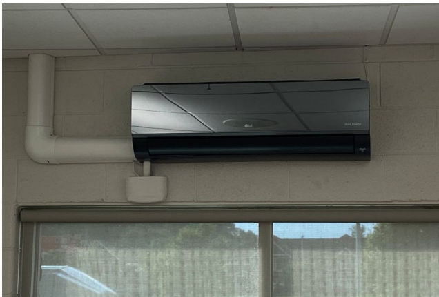
Classroom HVAC Unit
