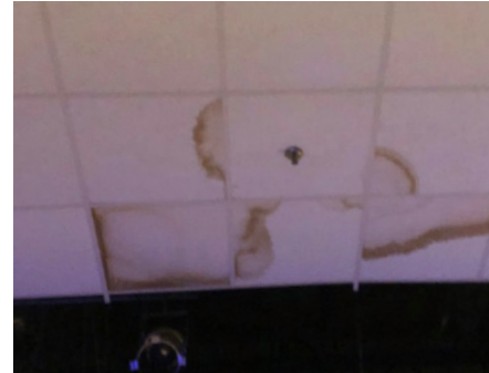
11 stains in ceiling tile
