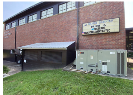
06 HVAC unit is exposed and within public view
