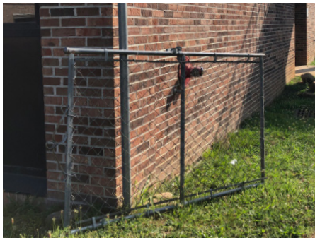
05 perimeter not secure; gate off hinges
