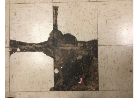
12 deterioration in VCT
