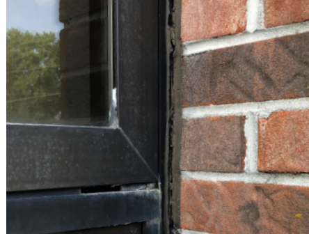
02 gap at window perimeter
