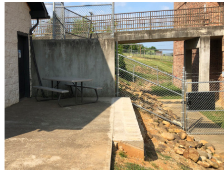
06 lack of safety barrier
