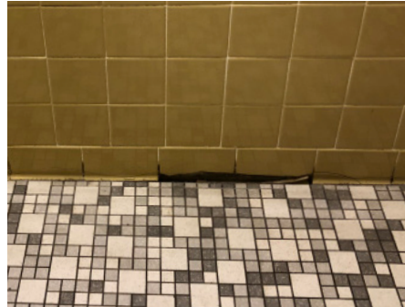
10 separation between wall and floor slab *
