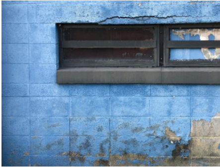
09 cracking masonry, peeling paint
