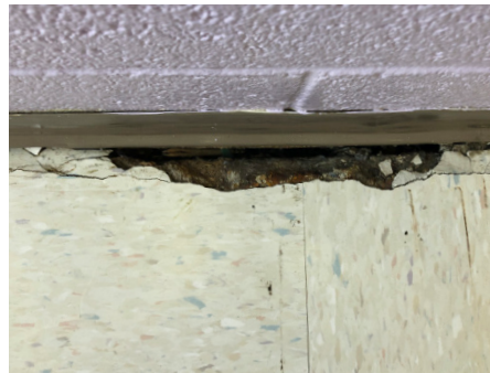
14 separation between wall and floor slab *
